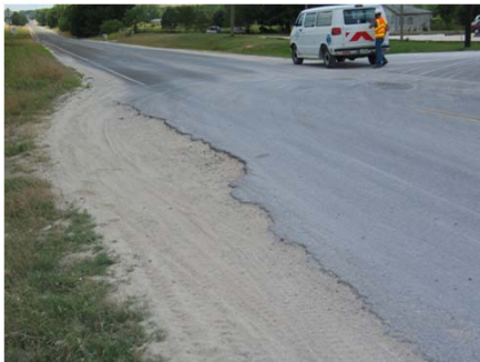
Tire tracks on unpaved shoulder
