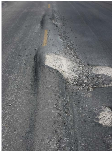
Pavement shoving, loss of surface
