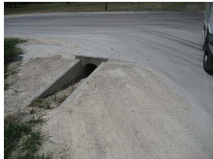
Tire tracks on safety end treatment
