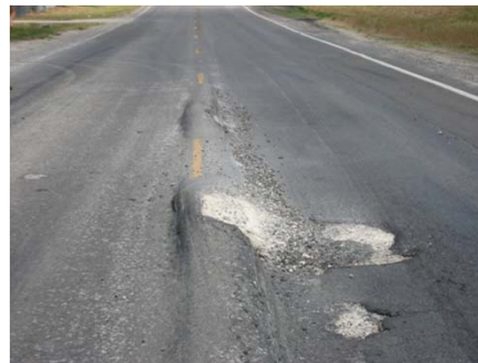
Pavement shoving, loss of surface
