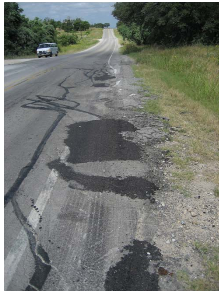
Shoulder patches, cracked seals
