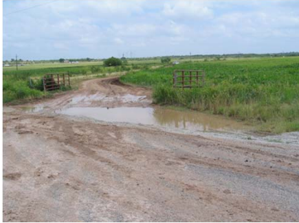
Drainage problem at driveway
