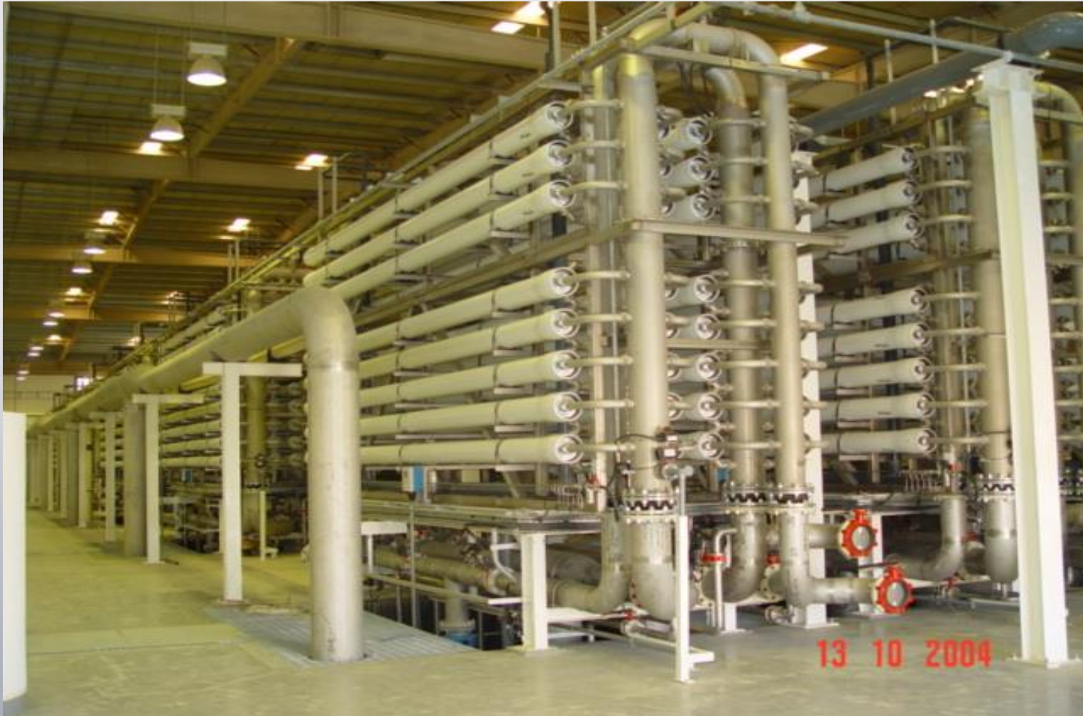
UF Skids and Piping
